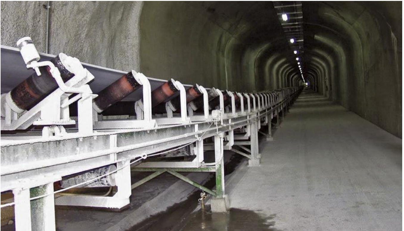
Immaculate conveyor tunnel at Hualien.
