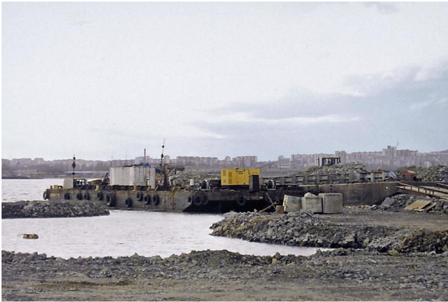
Atlas Copco generators are used on the Burgas port construction barges.
