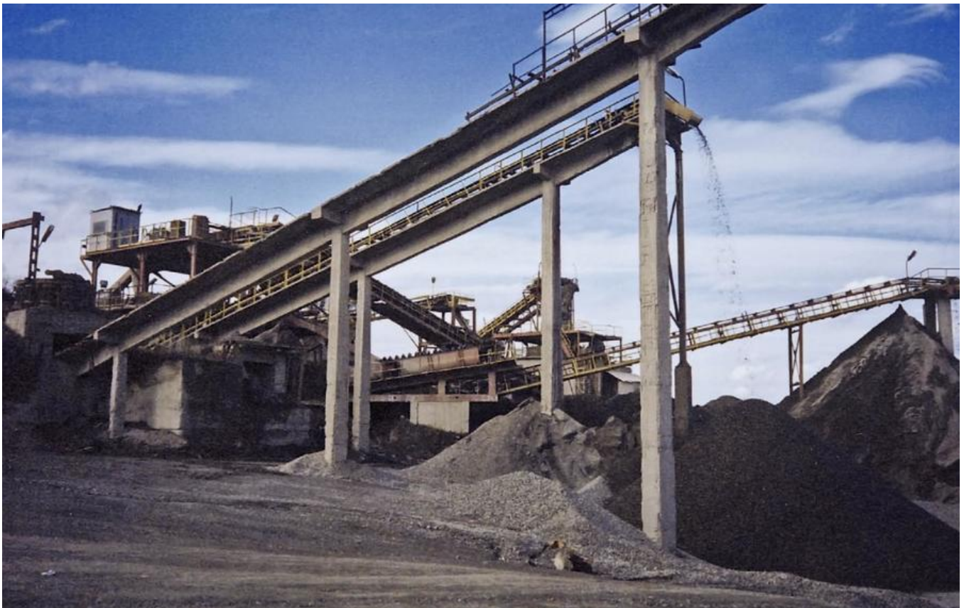
Crushing and screening plant at Andezit's Gorno Ezerovo quarry.
