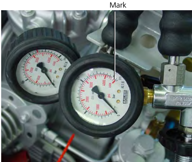
Abb. 33 Final pressure gauge
