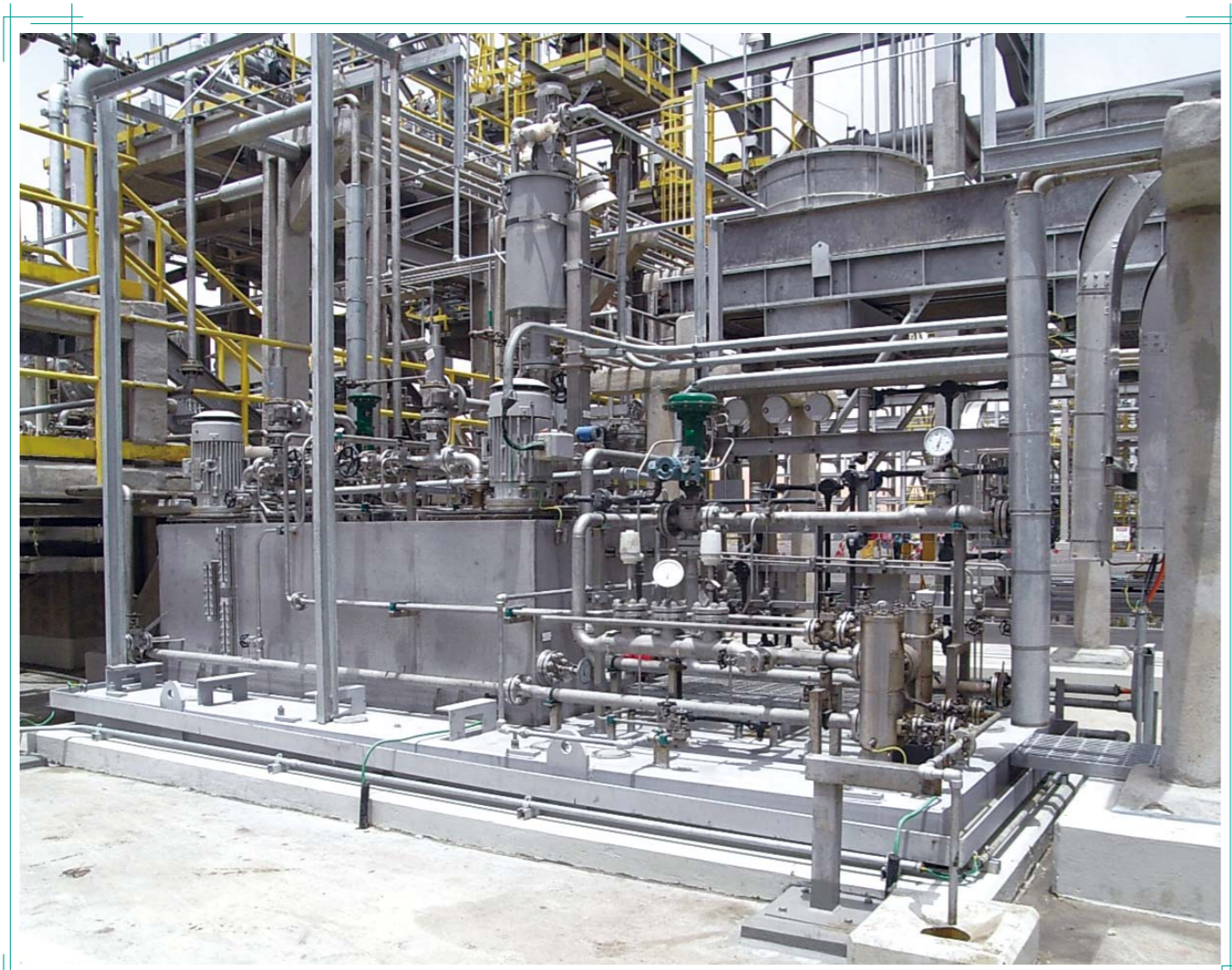
Lube Oil Unit
