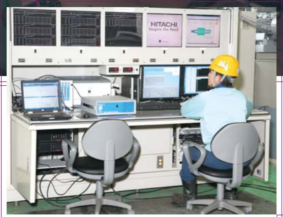
On-line Test Control Room
