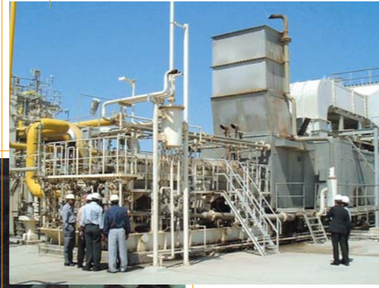
Gas Compressor for Gas Gathering Plant
