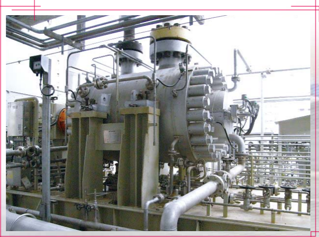
BCH506/B Injection Gas Compressor
