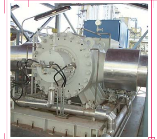
PCH601 Feed Gas Booster Compressor
