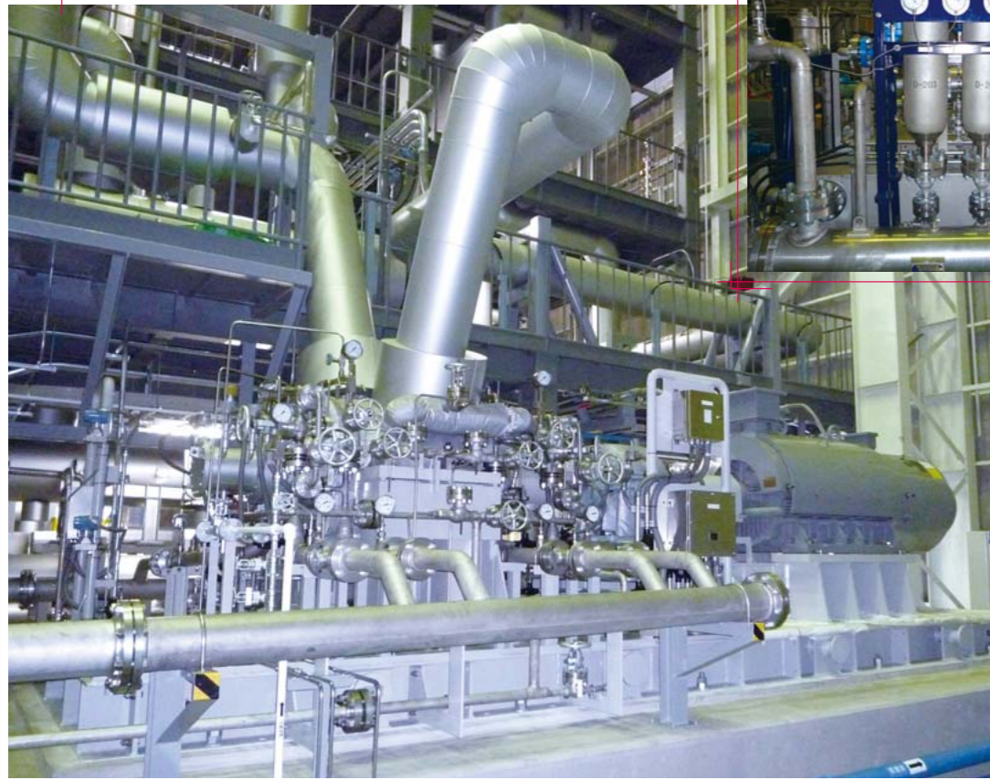
BCH301 Steam Compressor
