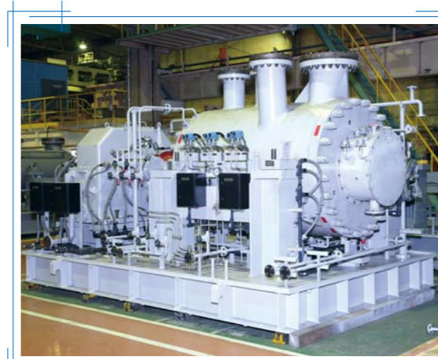
3BCH607 Propane Compressor
