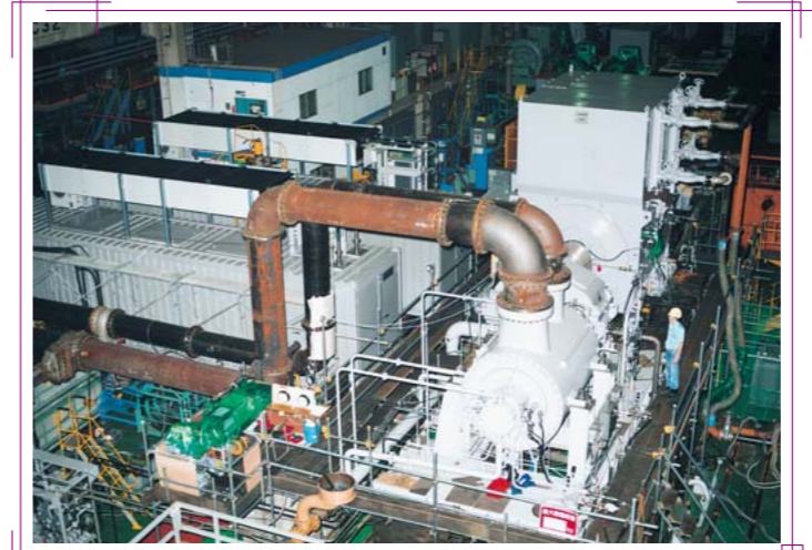
BCH804 Complete Unit Test with 35MW Motor
